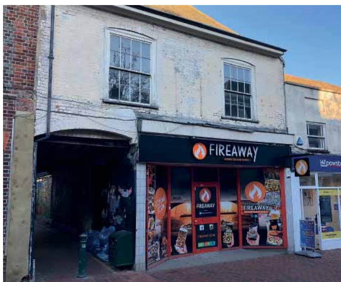
Degradation buildings in Sittingbourne High Street Conservation Area
